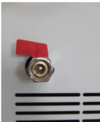
picture 1 drain valve
